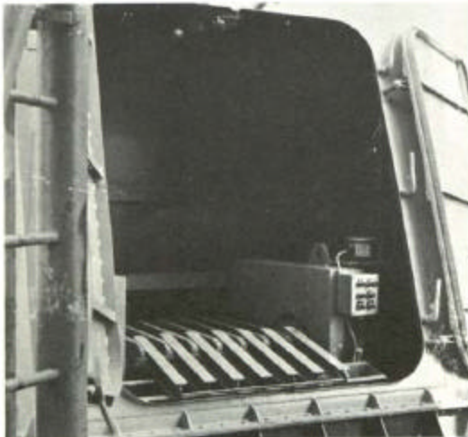
Top station 36A175 unit & deck house
