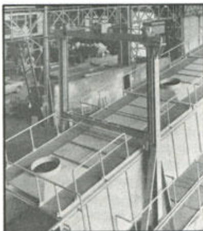
Flexible foam slab machinery
