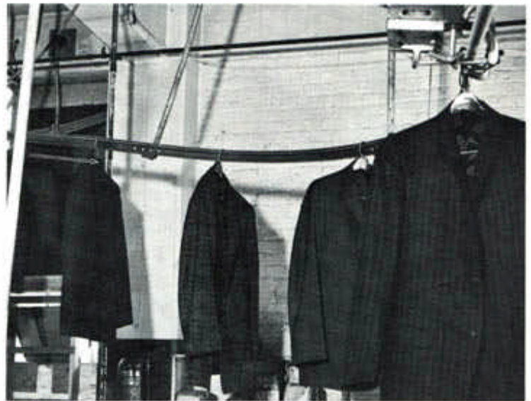
Monoflo Conveyor delivering garments from floor above to a slick rail. Automatic counter keeps record of the number of items transferred to the storage rail.
